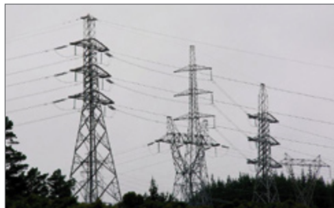
Photo 3: Transpower 220 kV transmission lines .
