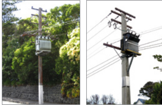
Photo 8: Example of pole mounted distribution substation (transformer).
