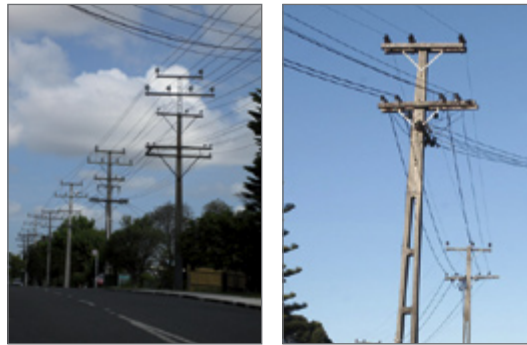
Photo 1: Examples of distribution lines with various layers. These examples include: 33kV on the top crossarm, 11kV on centre crossarm and 400V on bottom crossarm; 11kV on the top crossarm and 400V on the bottom crossarm. Structures often carry telecommunications including bundled fibre optic communications lines underneath the overhead lines .
