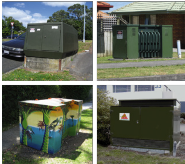
Photo 9: Examples of ground mounted distribution substation (transformer) often housed in purpose designed kiosks.
