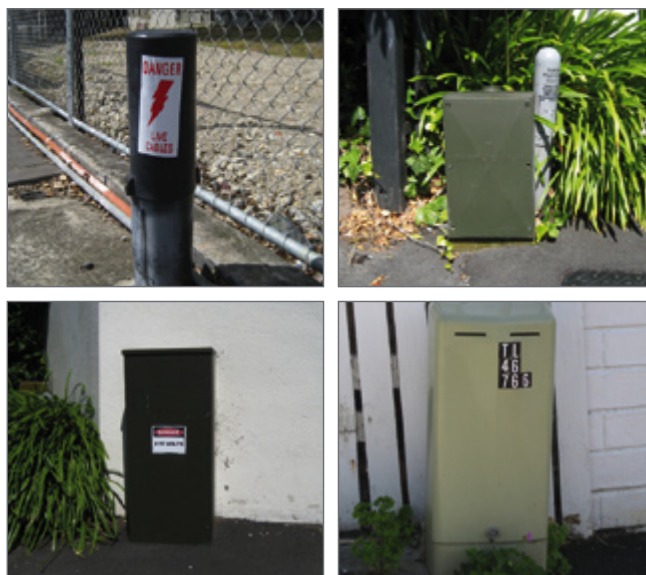
Photo 10: Examples of connection points, often referred to as ' pillars ' or ' plinths ', between the distribution network and the customer's underground electricity service (supply).
