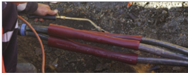
Photo 12: An example of a high voltage underground electric cable.
