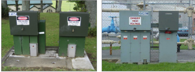
Photo 11: Examples of switchgear, used to connect or disconnect specific areas of the distribution network .
