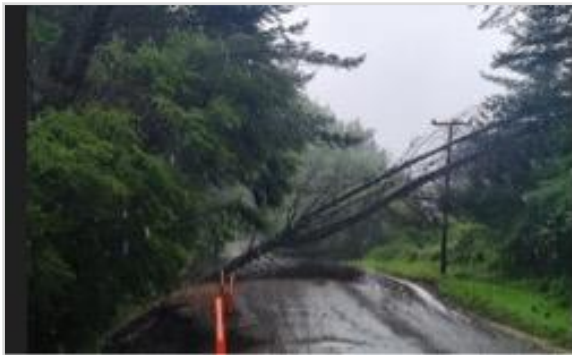
Figure 47: Line damage caused by trees outside the fall zone going through lines in April 2022
