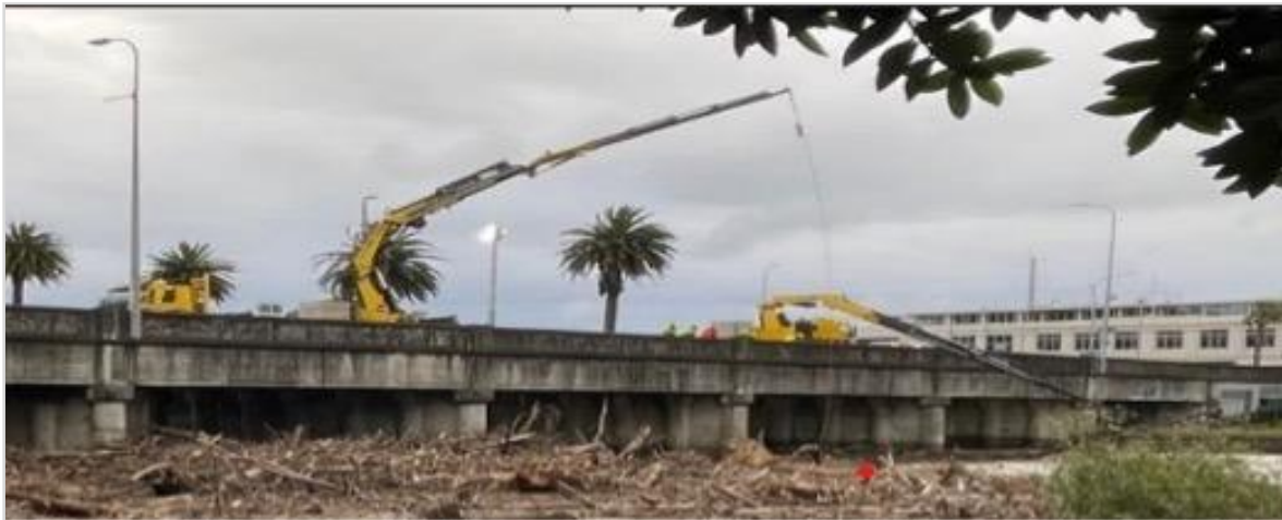
Figure 49: Damage to infrastructure in Tairāwhiti caused by floods in January 2022
